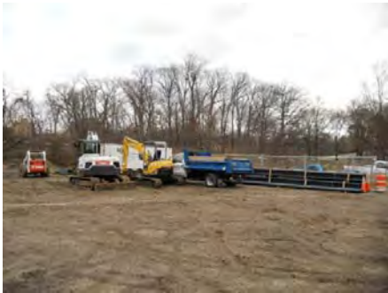
View of northeast corner of SMY where removal of impacted soil is proposed.
