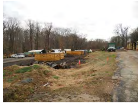
View of central portion of OWA looking west (areas where removal of impacted soil is proposed are on left and right side of photo).
