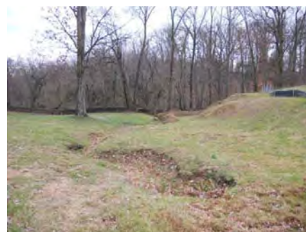
View of drainage feature located on northern side of SDS looking east.
