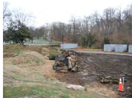
View of eastern portion of OWA used for storage of wood debris (former location of Building 107, areas where removal of impacted soil are proposed are on left side of photo).
