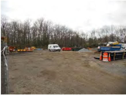
View of SMY looking west (area where removal of impacted soil is proposed is on right side of photo).
